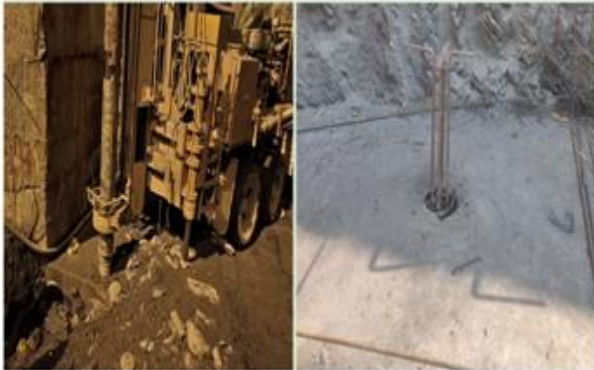
Fig. 5. Picture (a) Showing drilling equipment while drilling hole for micro-pile and Picture (b) Showing final micro-pile hole from top of the surface after complete reinforcement & concrete in Tehri PSP outlet foundation area.
