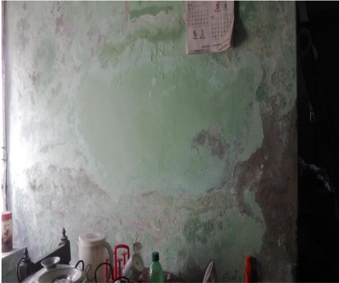
Fig. 14. A damp wall (Picture has taken from Sabujbag (Mugda))
