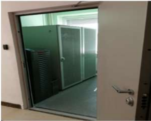
Fig. 2. Security door server, data, network center
