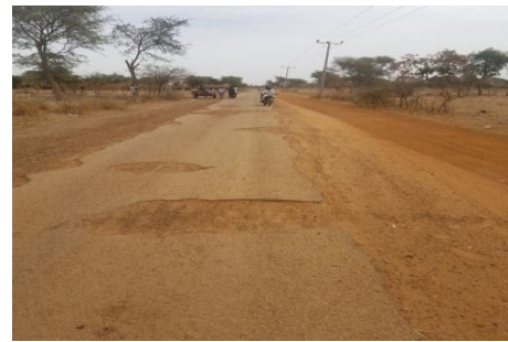
Fig. 3.2: Raveling (from visual site survey)
