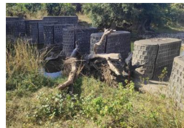
Fig. 2. Tree trunks and debris accumulation across the channel during flood season.
