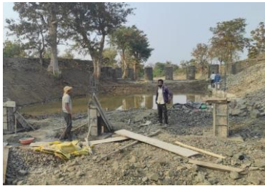
Fig.3. RCC columns newly constructed upstream to the KT weir for debris control.
