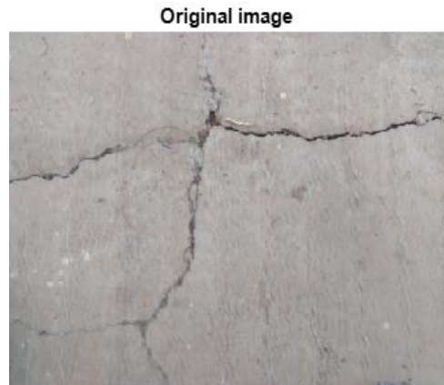
Fig. 7. Original Image of Road Crack.
