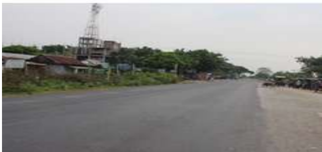
(a) No lane separated marking.
