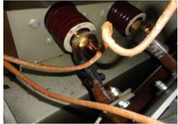
Figure 13- Faulty portion of bushing
