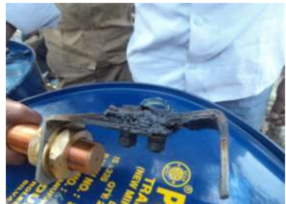
Figure 14- Damaged bushing clamp
