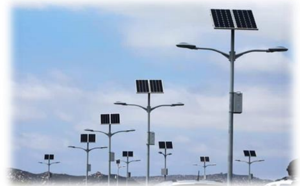
Figure 2: Solar panels on parking lights
